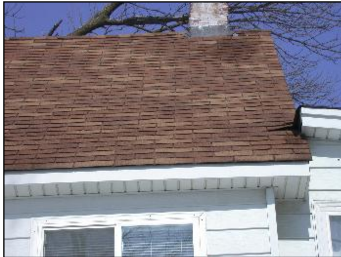
1. note lack of gutters
